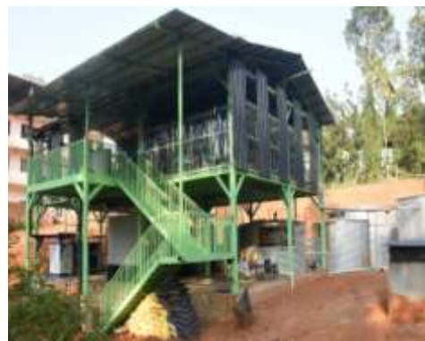
1 MLD STP at Kozhikode medical College
