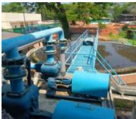
500 KLD STP at Kozhikode medical College
