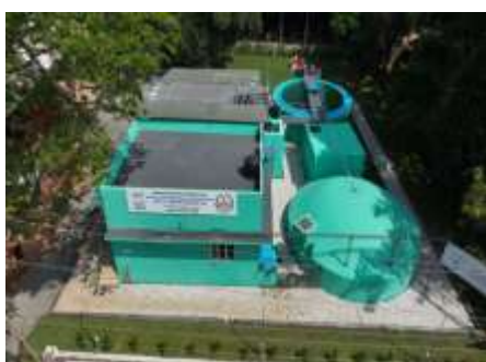
360 KLD STP at General Hospital, Thrissur
